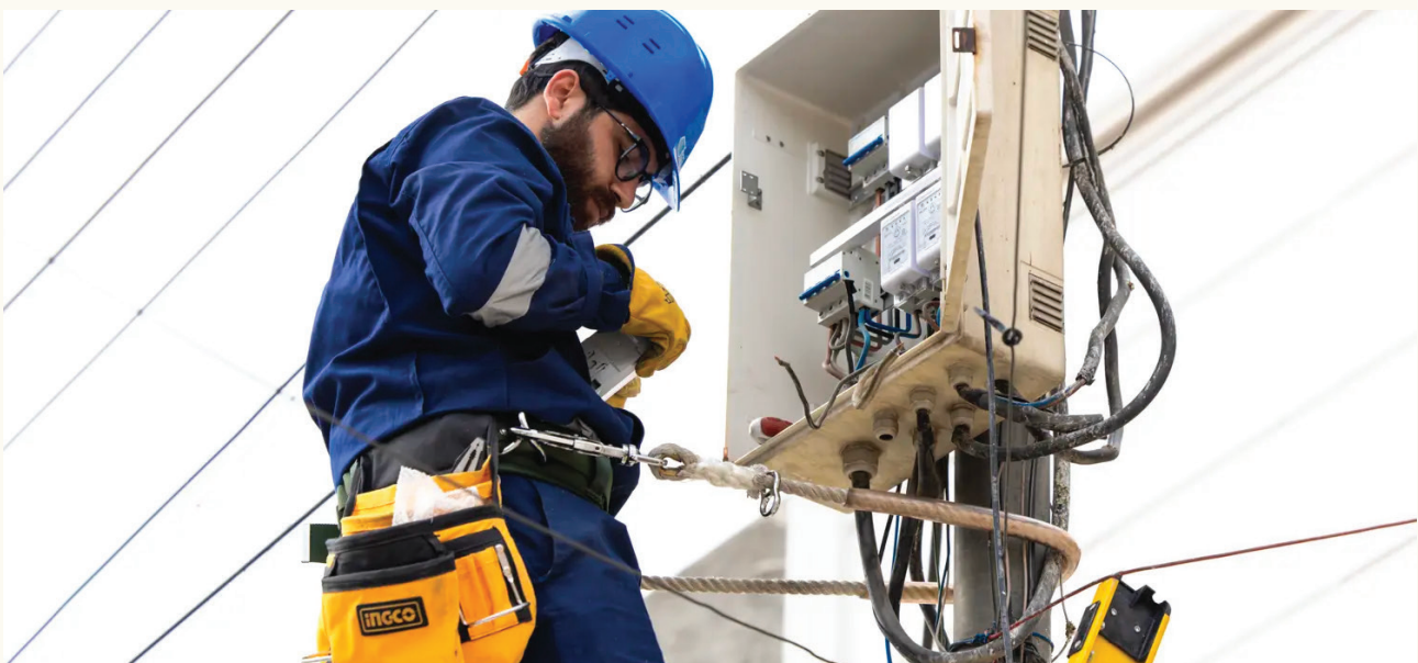
An electricity worker from KRG inspects a local neighborhood distribution board as part of the Runaki electricity program. Photo credit: Official Runaki Program website.
