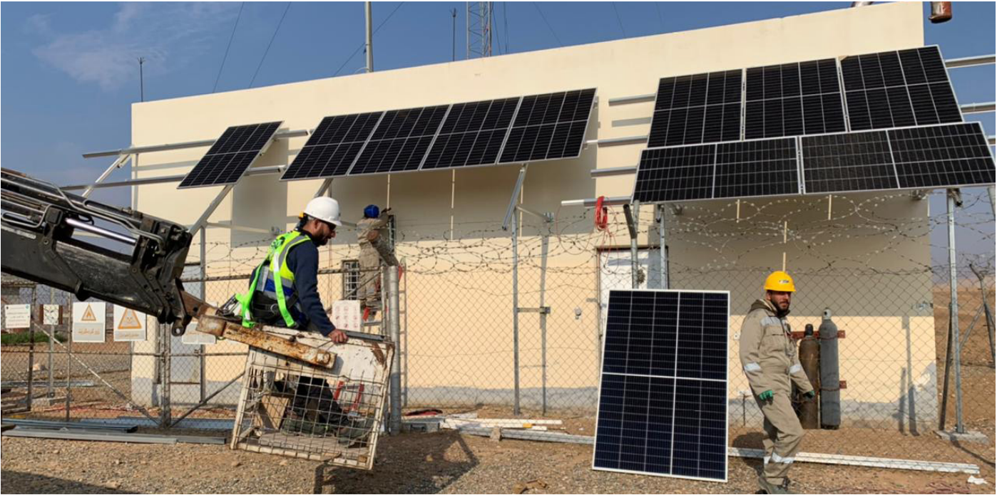
Installation of an off-grid wall mounted solar PV system in Chamchamal, Sulaymaniyah, 2021. Source: KESK
